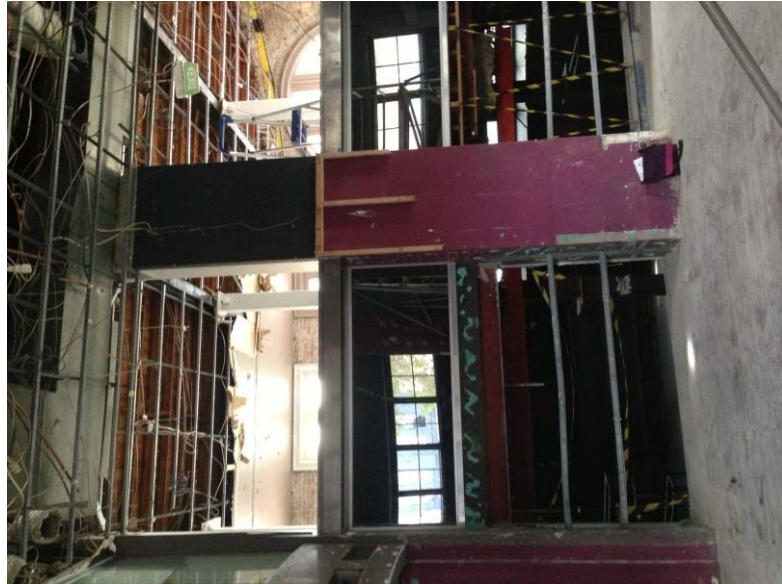
Lower ground floor level looking toward central structural spine and existing columns
